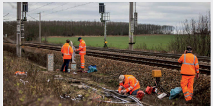
Sensor cable installation
