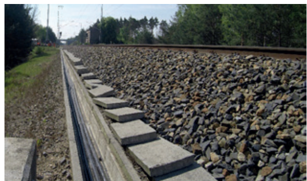
Fiber optic cable in duct along the tracks
