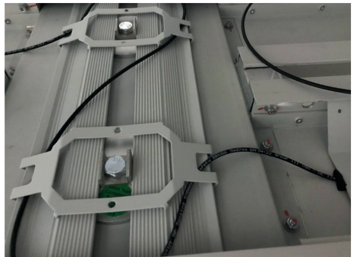
Figure 2: Sensor Cable on E&I 3200A bus duct joint
