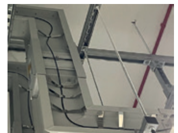
Sensor cable fitted on bus duct
