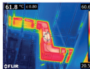
Thermal image of cable installed along bus duct
