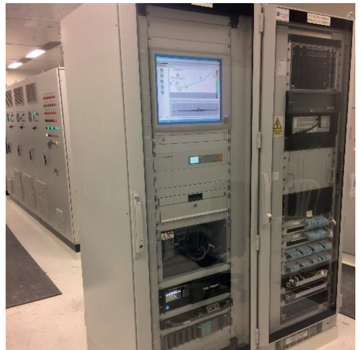
Figure 3: System installation and configuration
