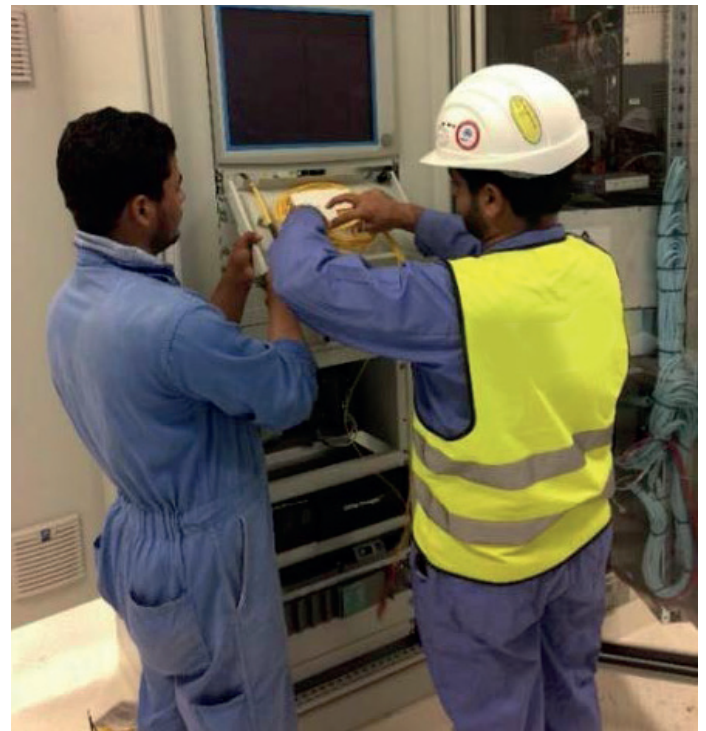
Figure 4: AP Sensing SmartVision in the remote control room
