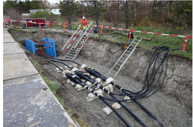
Figure 5: Three circuit phases for power cables (Copenhagen, Denmark)
