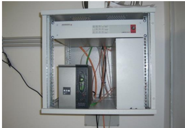
LHD instrument in the control room
