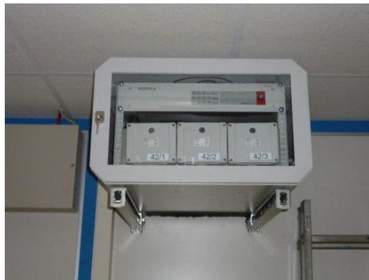
Linear Heat Series DTS device in operation
