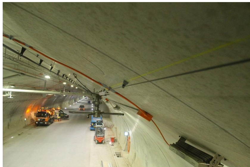
Sensor cable installed along the tunnel roof
