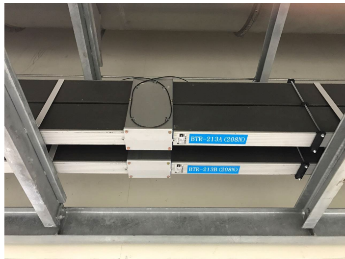
Fiber optic sensor cable installed on the bus duct
