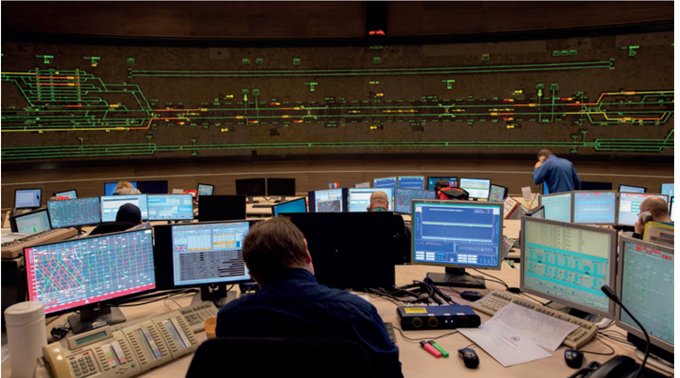
Figure 1: One of the two railway control centres (RCC), which monitor more than 36,000 different sensors installed in the tunnels. (Image: Eurotunnel)
