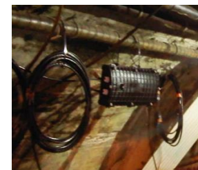
Splice box and ambient temperature measurement coil
