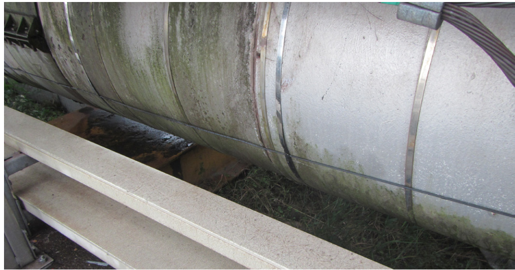
Fiber optic cable installed along terminal pipe
