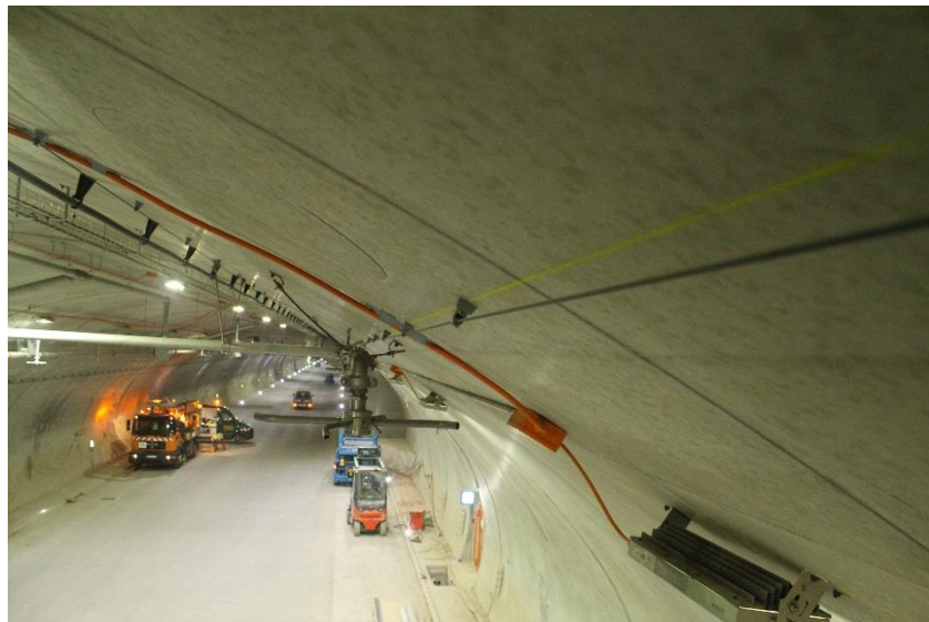
Sensor cable installed along the tunnel roof
