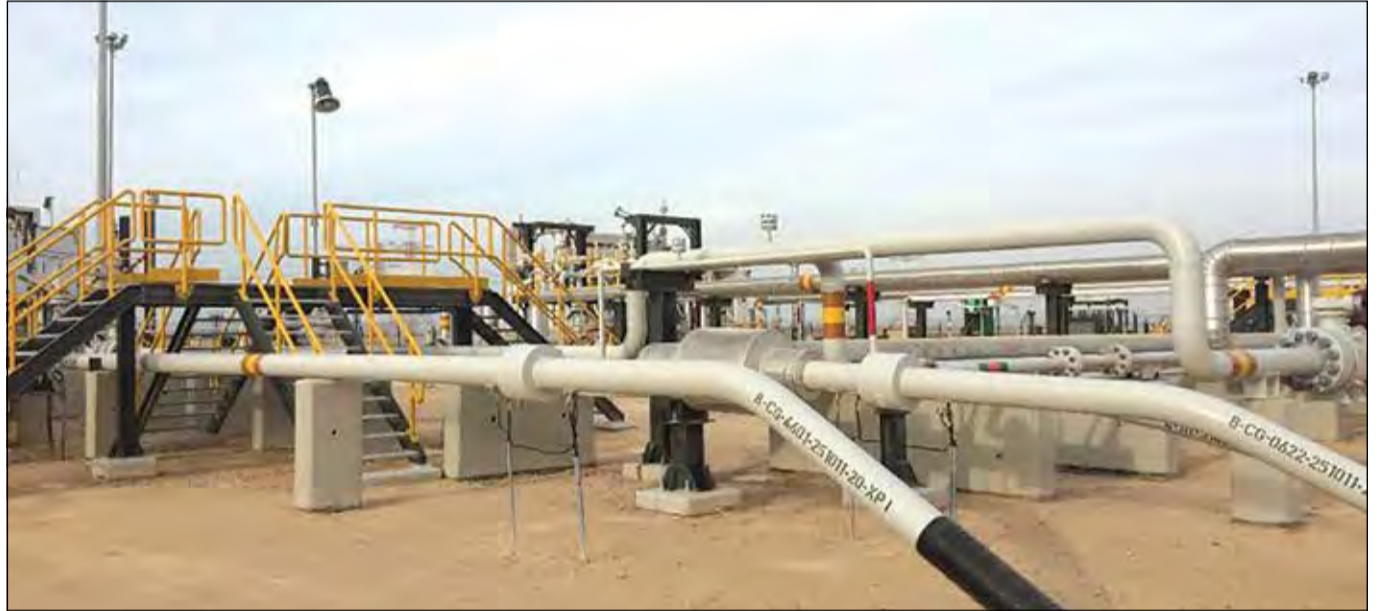
A CO 2 pipeline exiting the receiving station
