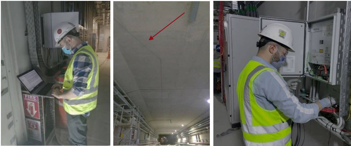
System Commissioning and Zone Configuration
