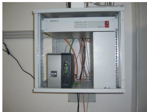
LHD instrument in the control room
