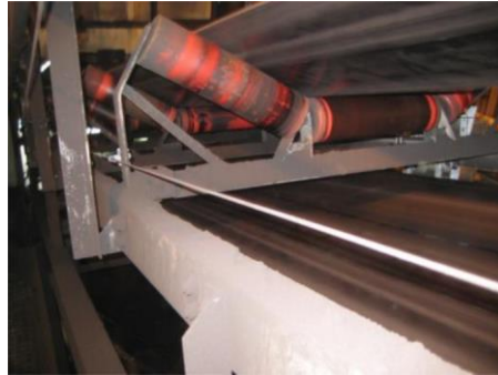
Figure-9: FO cable mounted on idler station of a trough conveyor
